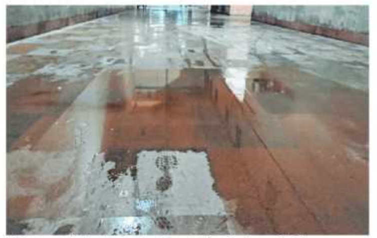
Water accumulated at Seawoods railway station after heavy rainfall
