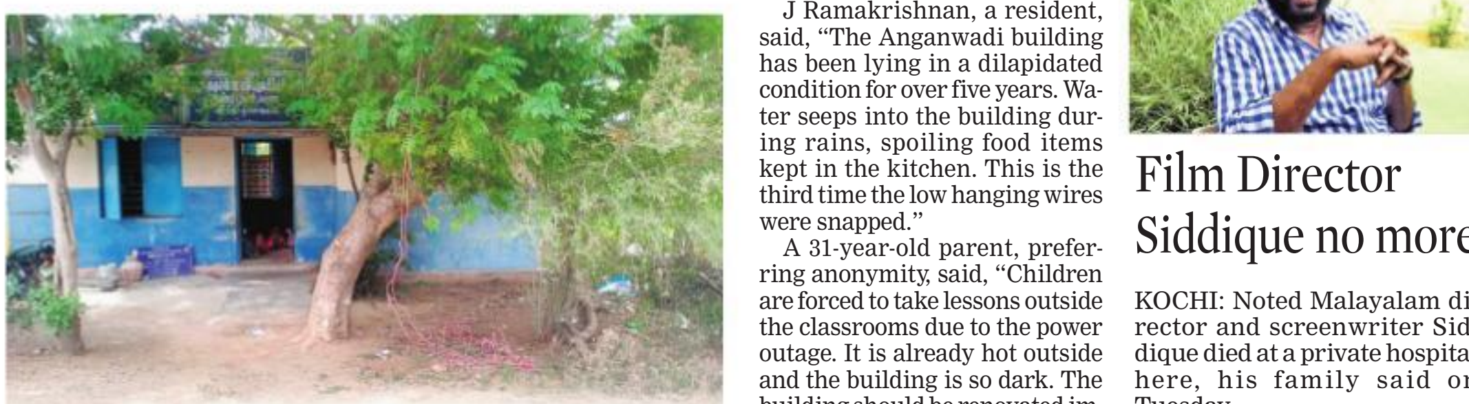
The Anganwadi centre building which is in a dilapidated condition | EXPRESS
